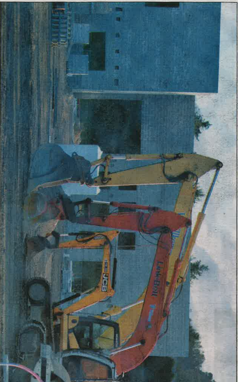
Construction crews work at the site of the Festival Foods in Hartford, 1275 Bell Ave.
